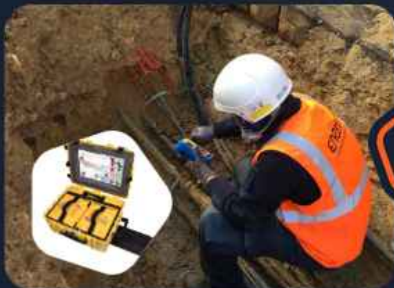
De-energized and dual grounded.
